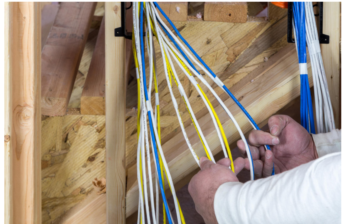
Keep the surround sound bundles together, like these TV/Data runs shown bundled together.
