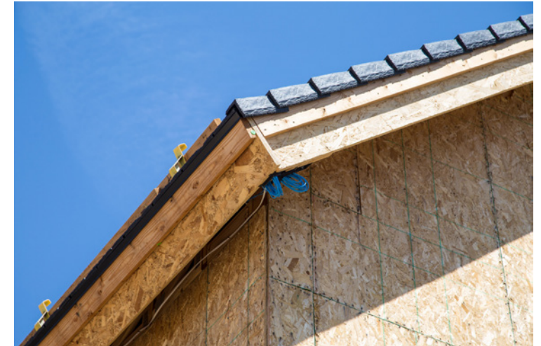
Surveillance prewire for 2 cameras.
