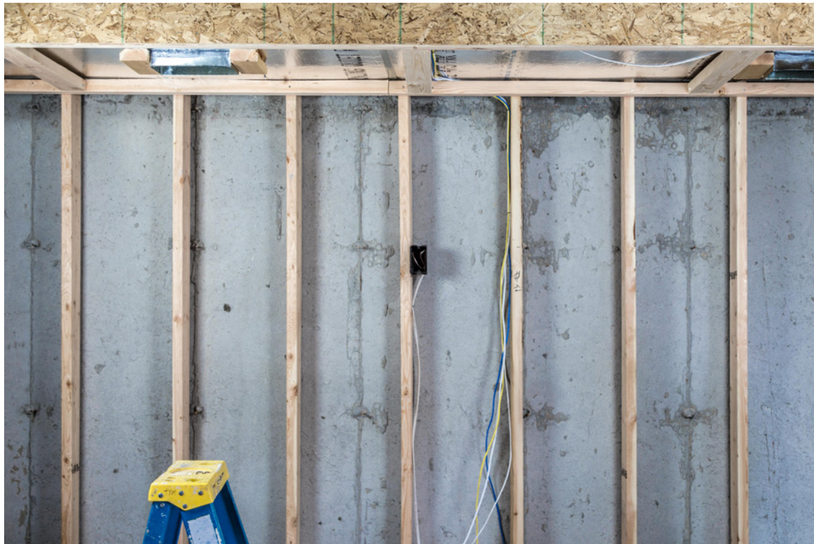
Untrimmed cables running along a stud.
