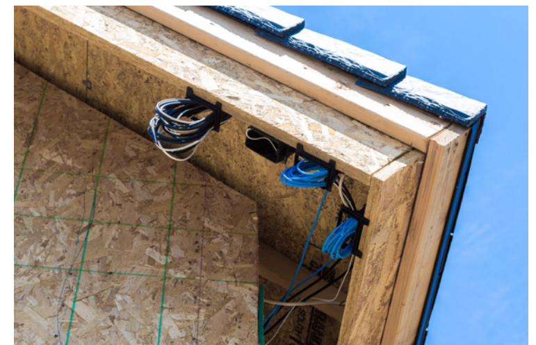
Satellite prewire bundle next to surveillance prewire.
