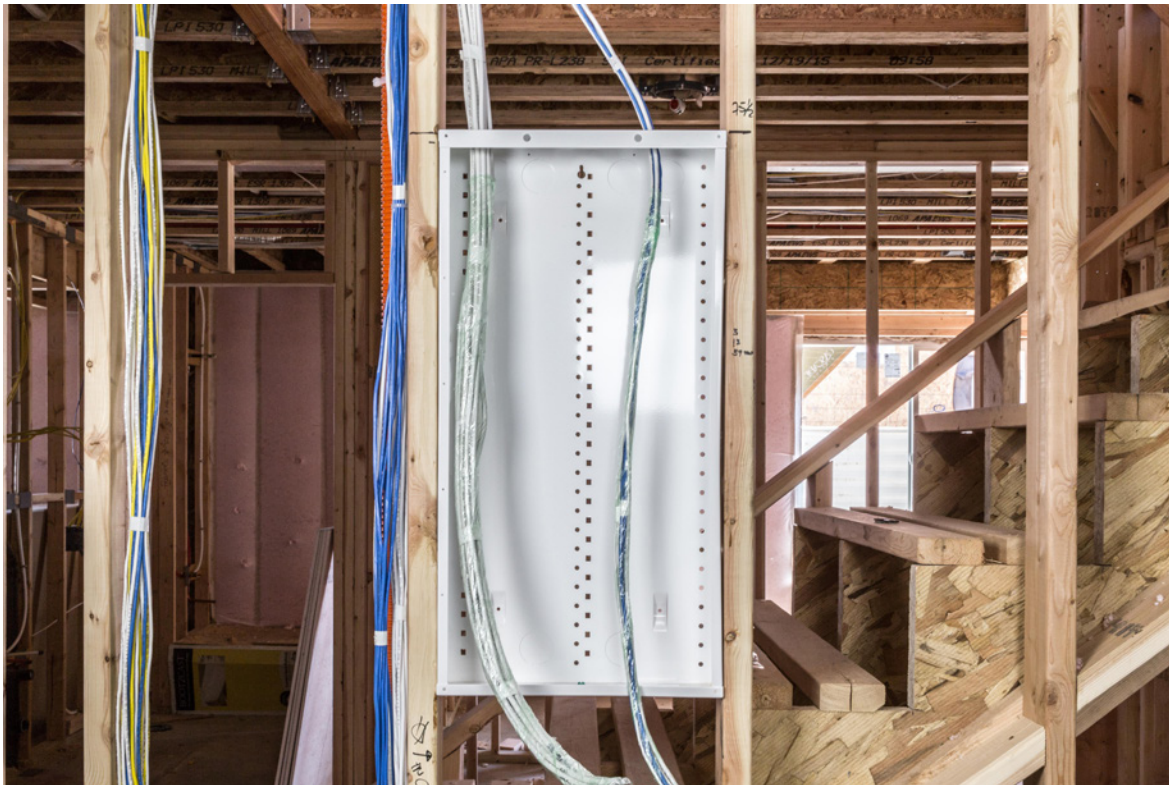
Low Voltage Can: Left side is for TV, Right side is for Coax
