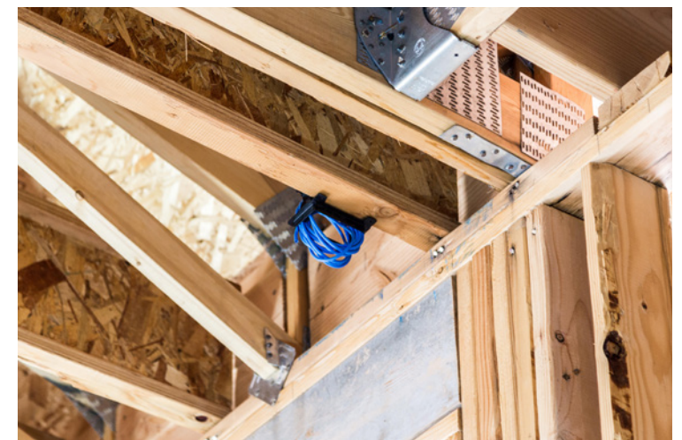
Indoor surveillance camera prewire
