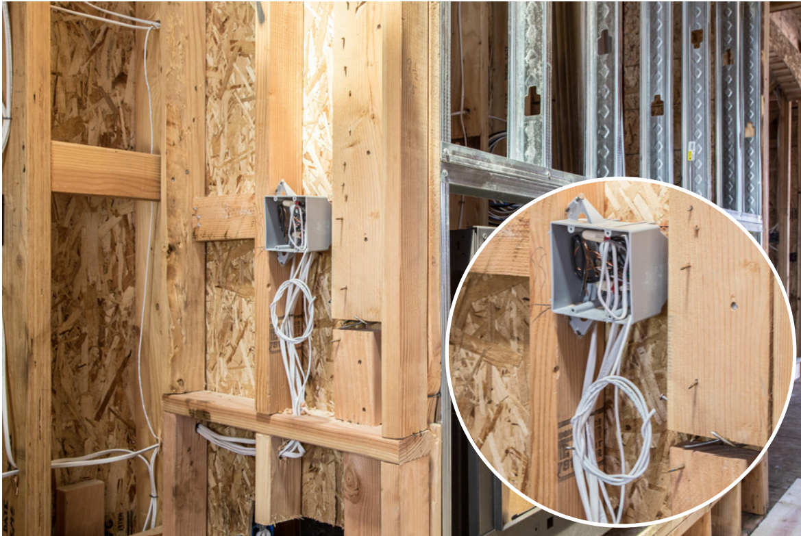
Fireplace control prewire.
