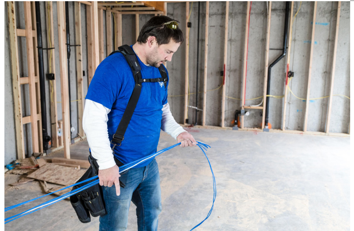
Keep all surround sound wires together.
