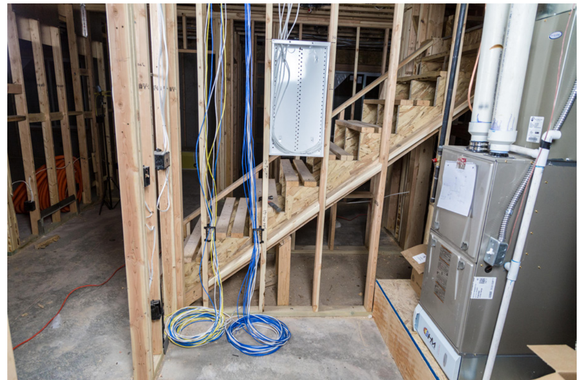
Always keep cable bundles tidy.
