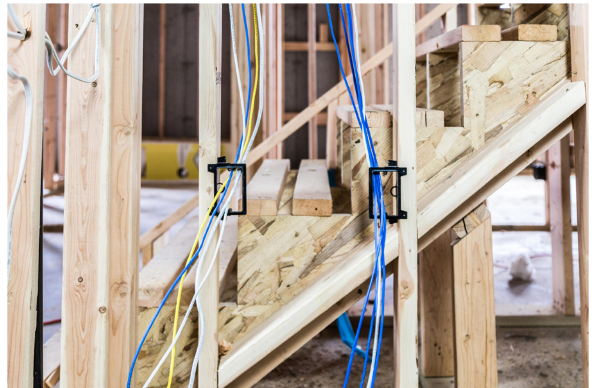
Low voltage brackets (mud rings) for the main snakes to the media rack.
